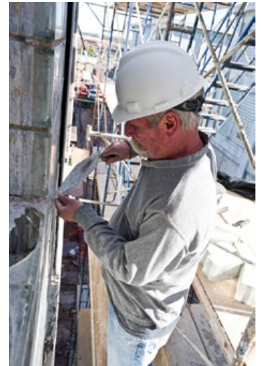
Individual restoration of glass blocks in former RJ Reynolds Tobacco company building
